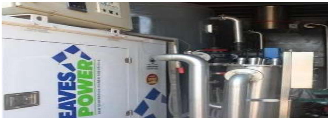
Figure 3: LWB Mobile Water Treatment Plant
